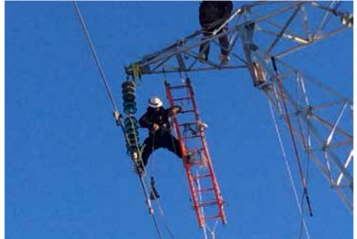
Crews replaced broken insulators on a 230-kv transmission line between the Teeland Substation and Point MacKenzie in February.
