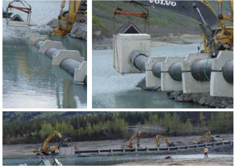
A siphon works will allow releases from the reservoir at Chugach's Cooper Lake Hydroelectric Project.
