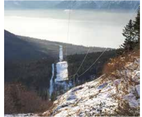
In preparation for a 2015 rebuild, crews cleared miles of transmission line right of way near Indian.
