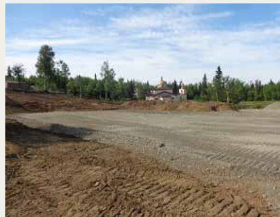
Chugach is building a new distribution substation on the Hillside. The facility, named the Hane Substation, is under construction at the intersection of Hane Street and O'Malley Road, east of Lake Otis Parkway. The $10.9 million project is necessary to meet the growing demand for electricity in the area. Site preparation began in July and construction will continue into 2016.
