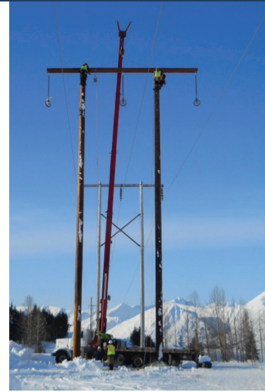
Work has continued throughout the winter on a rebuild of 15 miles of the transmission line linking the Kenai Peninsula and Anchorage.
