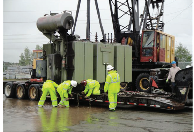
Crews have been moving material into the new Operations storage yard at the headquarters complex. Chugach built the yard to store equipment that was formerly on the site that will be used for construction of the new Southcentral Power Project. Per regulations, oil filled equipment like the power transformer in the photo will be stored in a location equipped with an oil containment basin.
