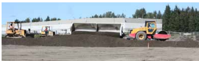
The contractor has established the base and grade of the SPP site
