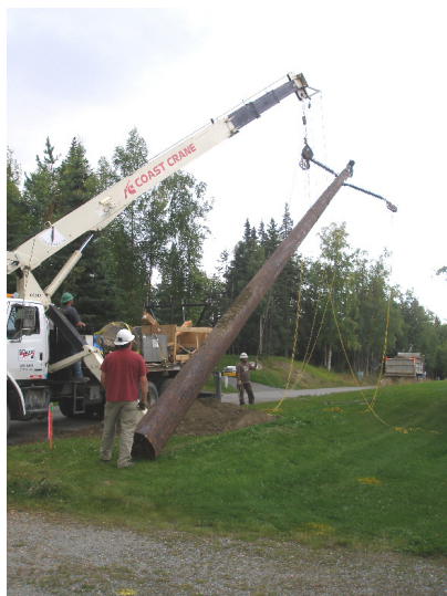
A wood structure is raised along Elmore Road as part of a project that will ultimately link three Chugach transmission substations in Anchorage. A transmission line project along O'Malley Road planned for 2009 will complete the 138-kilovolt loop between the Retherford and University substations.
