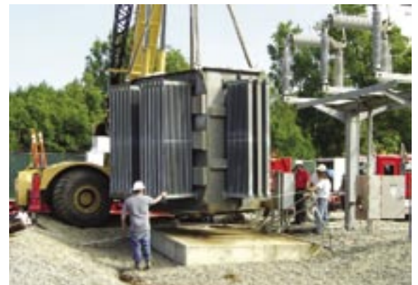
Chugach crews guided the reactor as it was moved from a concrete pad in the Pt. Woronzof Substation to a truck that brought the piece of equipment to Chugach's operations yard earlier this year.
