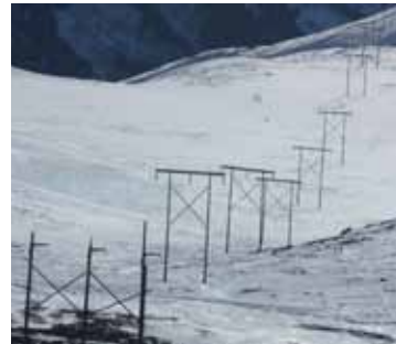
115-kv line crossing Powerline Pass
