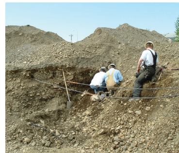
Workers try to locate a third cable after finding other damaged cables.
