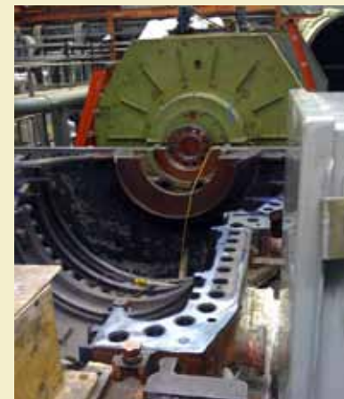
Crews at the Beluga Power Plant have dismantled Unit No. 8 for an annual inspection.
