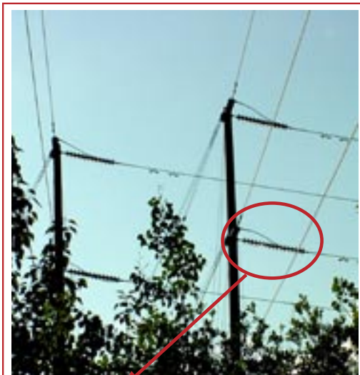
This new insulator string on a transmission structure along the Glenn Highway replaced one that shattered at the start of a major outage.
