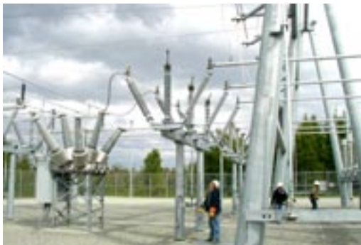
South Anchorage Substation
