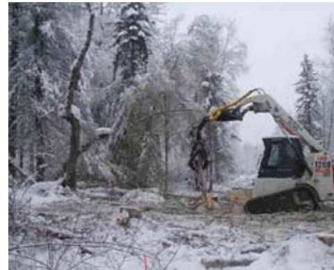
Relocation project: Chugach cleared a 30-foot right of way along the Hope Highway as part of a 1.5 mile line relocation project. The project will improve reliability, shorten outage time and lower maintenance costs by moving a section of difficult-to-maintain line from deep in the forest to a new alignment along the highway.
