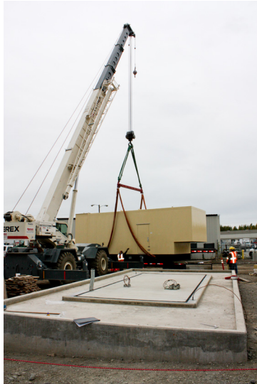
The new power plant's black start diesel generator package being set onto its foundation
