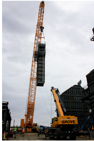
Alaska Crane's 600 Ton crane lifts the last large boiler assembly into place for SNC Lavalin
