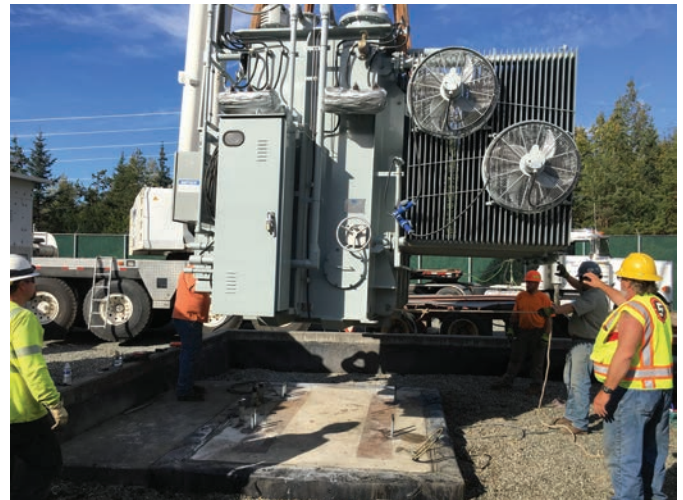
A new substation transformer was installed at the Baxter Substation.
