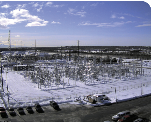
Top: The International Transmission Substation ties the new Southcentral Power Project to the grid.
