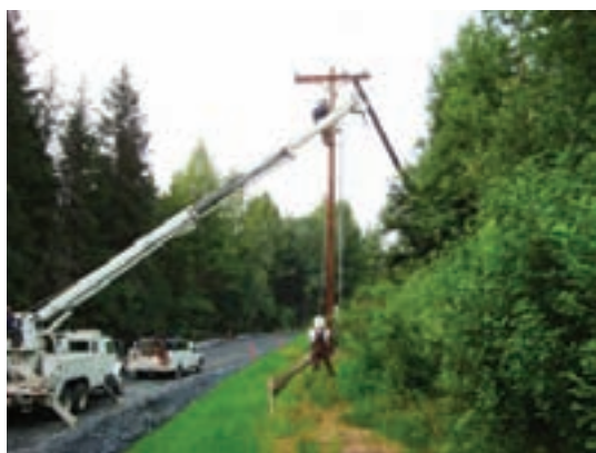
Chugach crews relocated overhead lines for a Department of Transportation road improvement project along Crow Creek Road in Girdwood.
