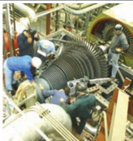
Chugach performed a major overhaul of Beluga Unit No. 8, a steam unit that is fueled from the waste heat from Unit Nos. 6 and 7.
