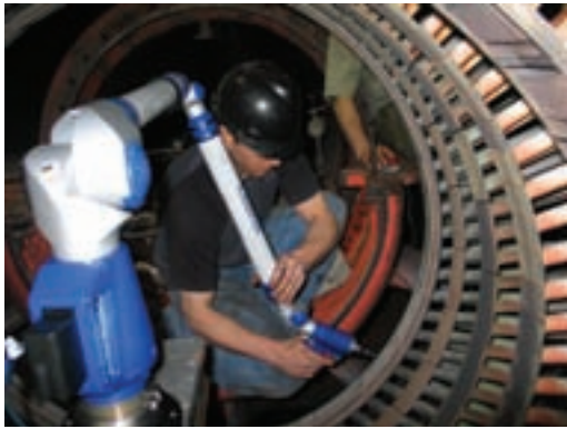
Chugach crews performed an internal alignment on the gas turbine of Beluga Unit No. 7 during a major overhaul of the unit.
