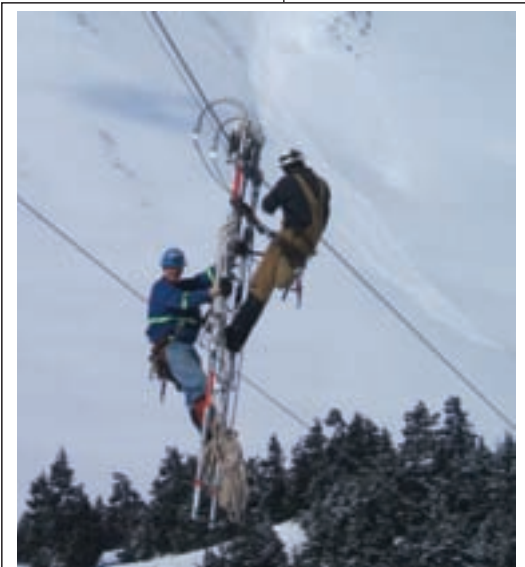
A Chugach crew installed new aircraft warning balls on the 115-kilovolt transmission line in Turnagain Pass.
