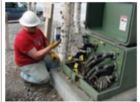
In 2008 Chugach budgeted $450,000 for cable injection projects including Towne East, International Square and Highland Park subdivisions.
