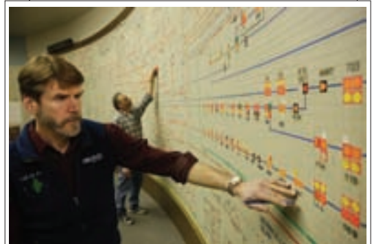
Chugach's SCADA system is a critical component of its Power Control Center.
