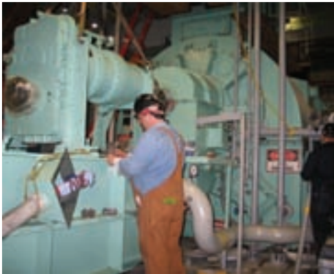
Chugach crews performed a major overhaul on Unit No. 7 in 2008, one of the two largest units at the Beluga Power Plant.
