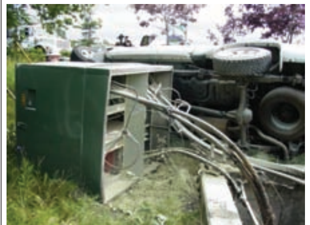
Chugach bills for damages to its facilities.
