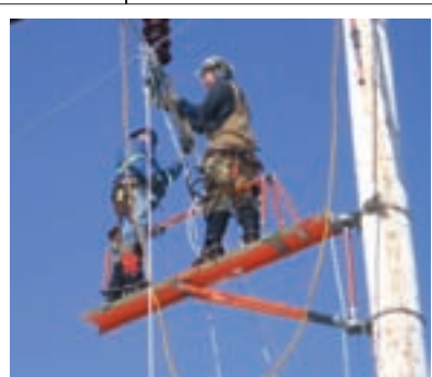
Chugach crews performed maintenance on the 115-kilovolt transmission line in Turnagain Pass.
