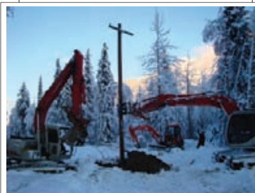
Chugach relocated a portion of the distribution line along the Hope Highway.
