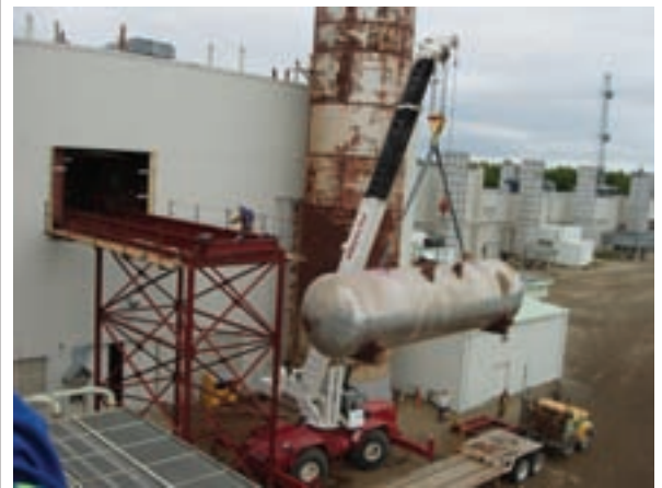
Chugach removed an old deaerator unit, which removes air from steam, during the 2008 Beluga Unit No. 8 major overhaul.
