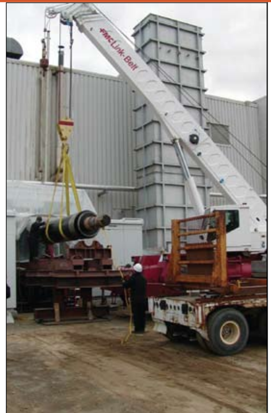
▲ Chugach crews moved the generator rotor into the building where it was reinstalled into Unit No. 5 during its inspection and rebuild.
